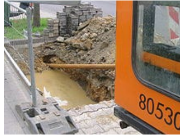
Starting pit with pilot hole and some drilling fluid in the pit.
